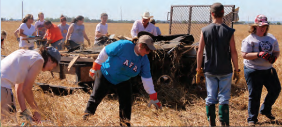
AFR/OFU volunteers, including Director Mike Humble, load debris during the "Field of TEAMS" event.
